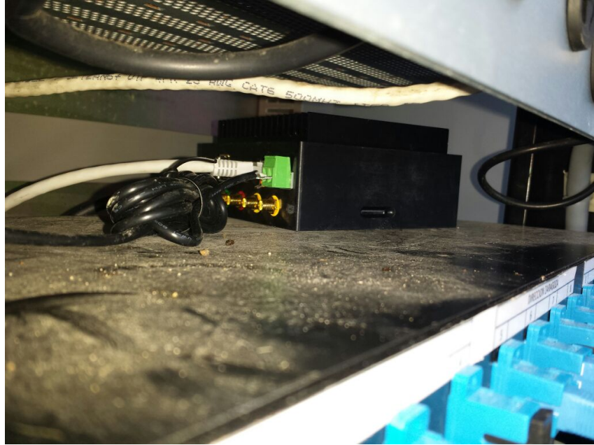
Figure 8: Access router connected in a roadside ITS-S in the A-2 highway
