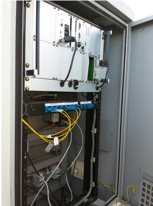
Figure 7: Interior view of a roadside ITS-S in the A-2 highway
