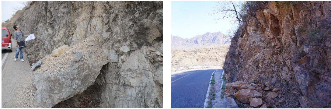
Figure 2. Rockfalls at the Zhenluoying area of the study area (photographs were taken on April 2013).
