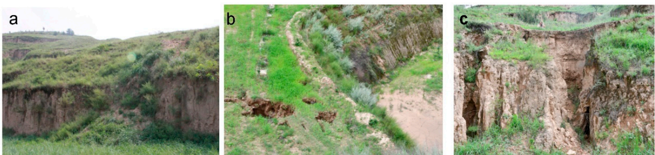
Figure 1. Terrace damages found by our field investigation. The damages generally include (a) collapse; (b) terrace sinkhole; and (c) ridge sinkhole.
