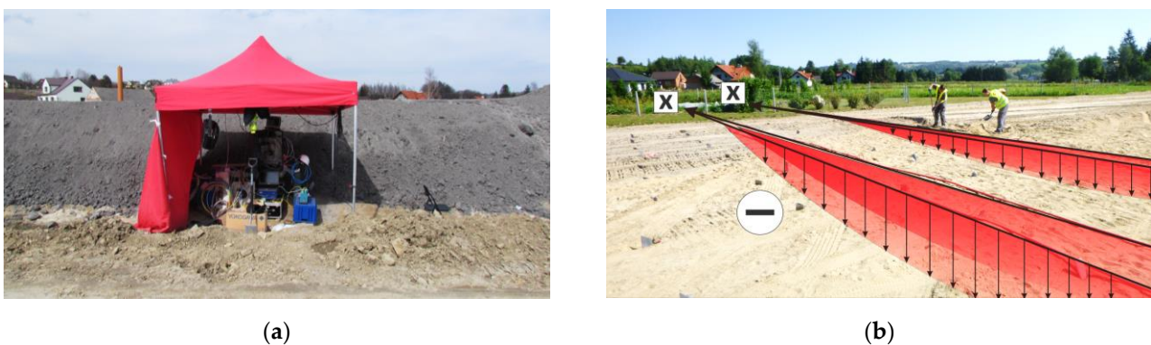
Figure 18. (a) The view of station next to the slope of embankment during one of the measurement sessions; (b) visualization of predicted displacement profiles with assumed signing (negative values correspond to downward displacements).
