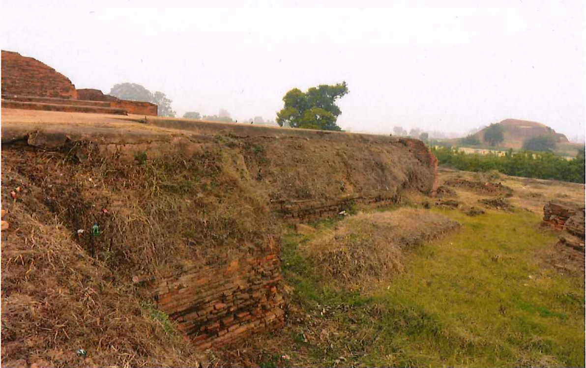
Structural Conservation at Temple site 13 (before)
