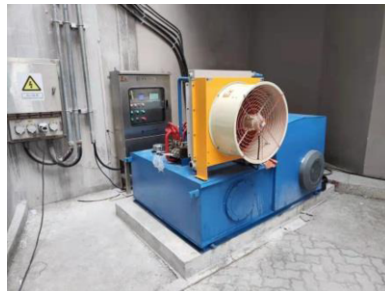
(2) Hydraulic Pump Station
