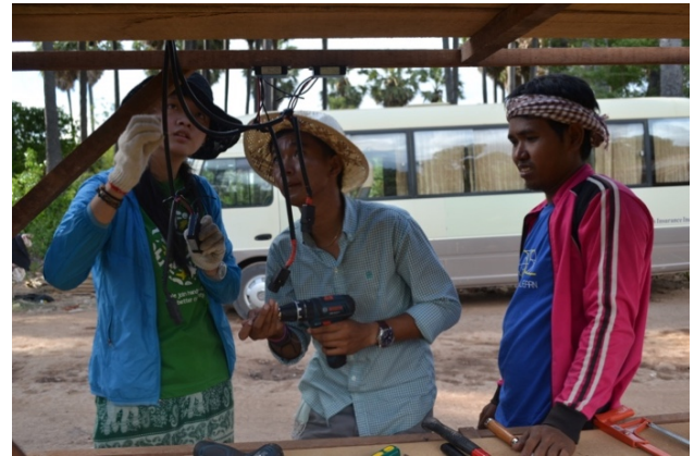
Fig. 3. A student from Faculty of Business was teaching a local volunteer to install a solar controller on the charging station
